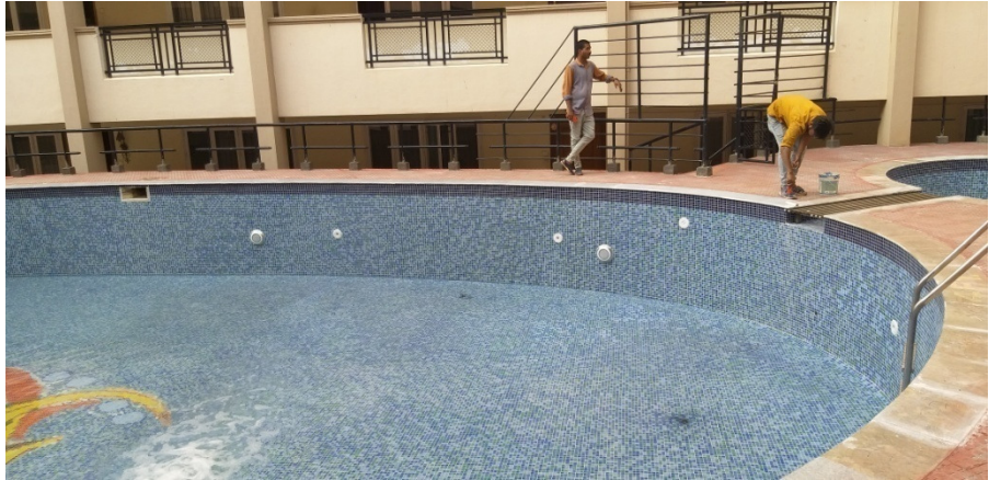
Underwater Light Fixed to Wall
