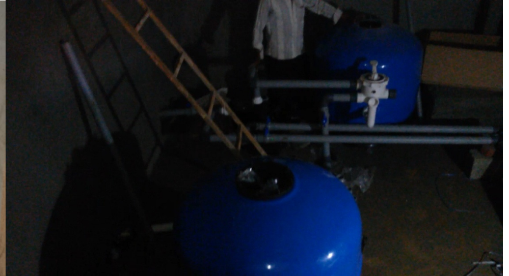
Filtration Room Setup
