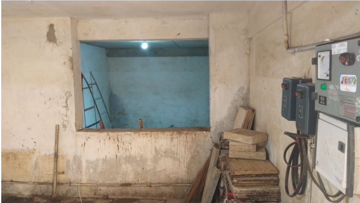
Filtration Room Electrical Control Panel Setup
